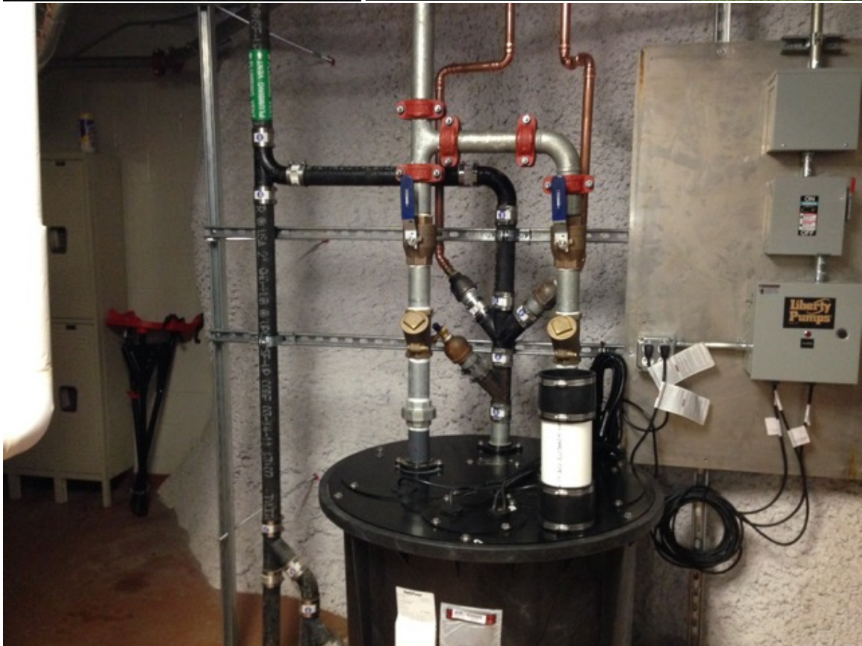
Above: Booster pump for current bathroom system.
