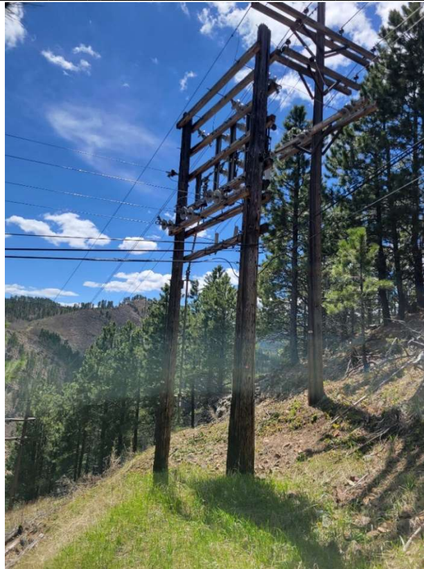
Figure 1. Picture of first pole structure that was visited during site visit (Pole #88).
