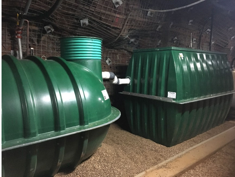
Figure 1. Davis Campus Wastewater Treatment Plant
