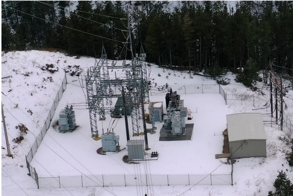
Figure 5.1 - Oro Hondo Substation
