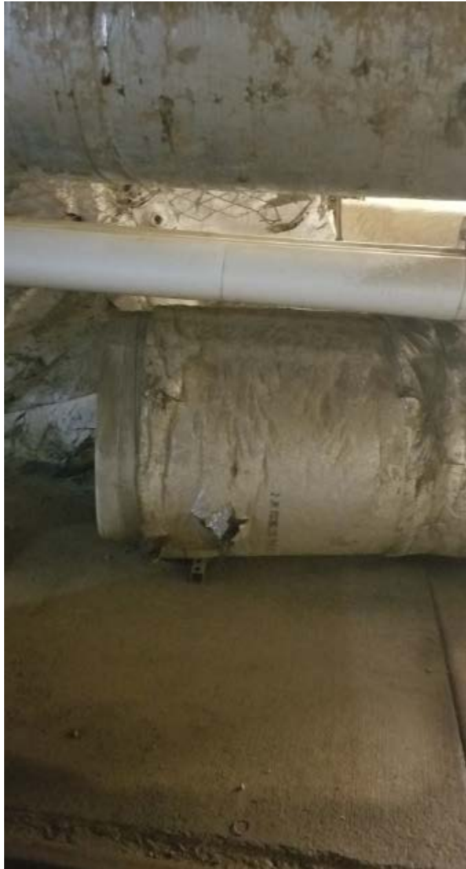
Figure 1. 32-inch Exhaust Duct for AHU-6
