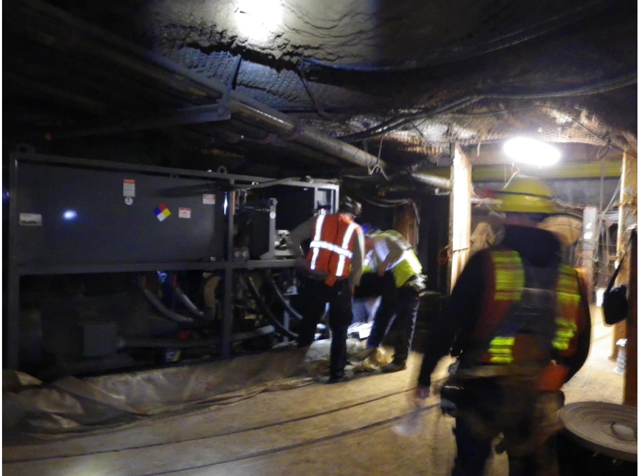
#4. HYDRAULIC POWER PACK ON 4550L
