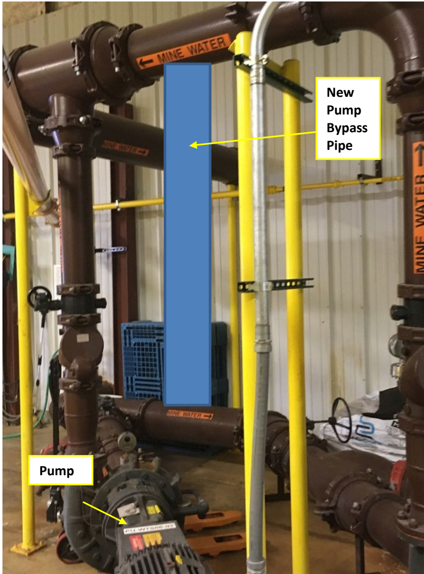
Attachment F.4 Pre-treatment (Yardney) Pump bypass – front view
