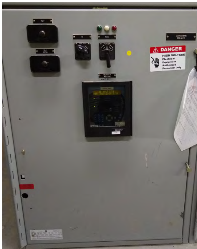
MAIN CB Section Front View
