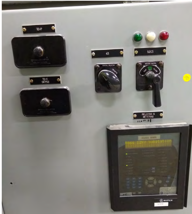
MAIN CB Section Front View
