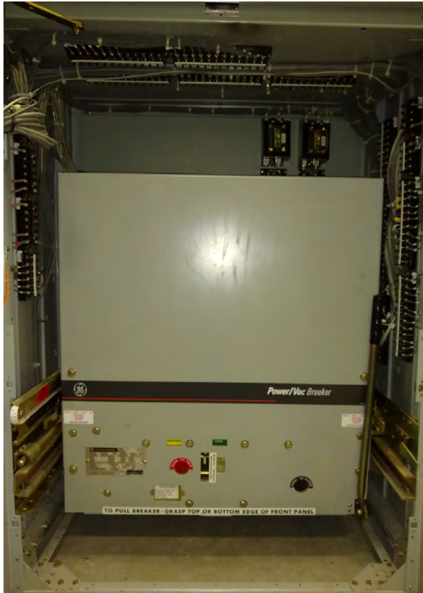
MAIN CB Assembly Front View
