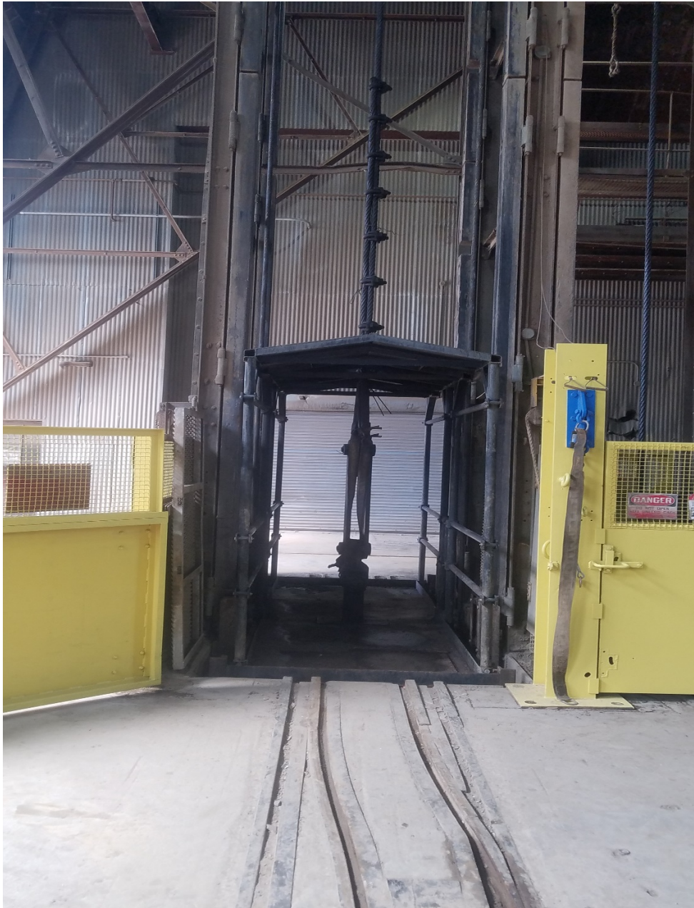
Photo #1: Yates South Cage Bonnet area with Thimble attachment to hoist rope.
