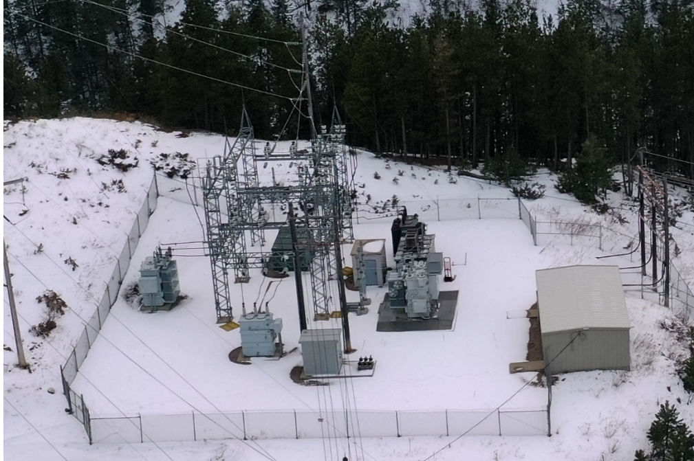
Figure 5.1 - Oro Hondo Substation
