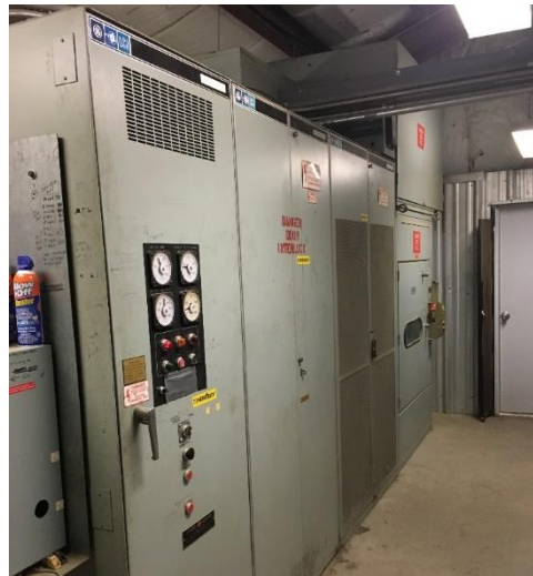
Figure 2 Current 3,000 HP VFD
