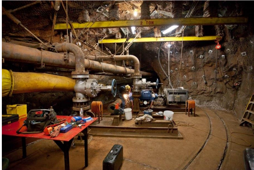
Figure 2. Photo of the Pump Room on the 5000L
