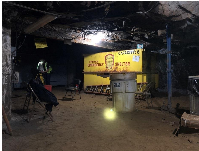
Figure 3. Outdated 6 Man Refuge Chamber at the 2450
