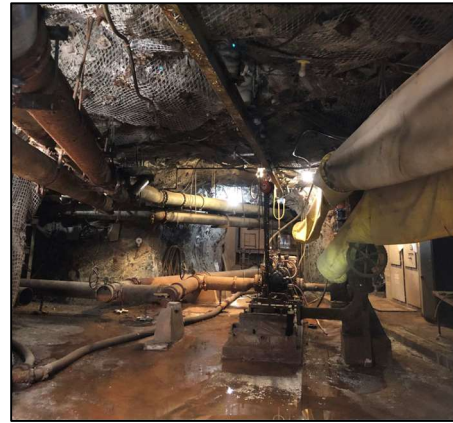
Figure 3. 3650L Pump Room
