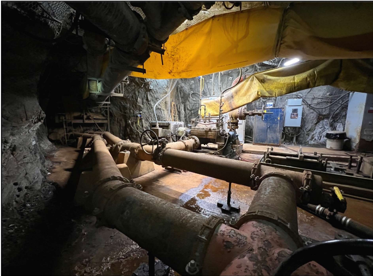
Figure 1. 3650L Pump Room
