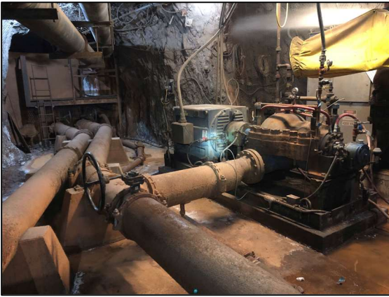
Figure 2. 3650L Pump Room
