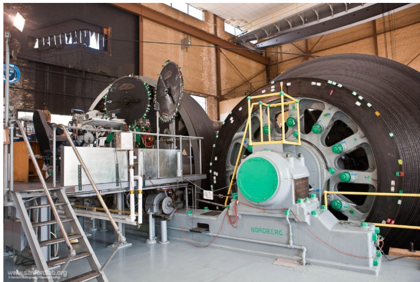
Figure 1. Ross Cage and Counterweight Hoist Rope Drums
