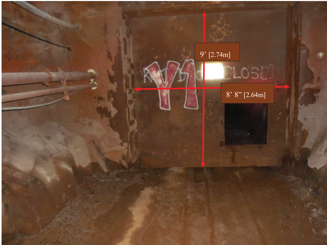
Figure 25: West Drift Access Vent Door
