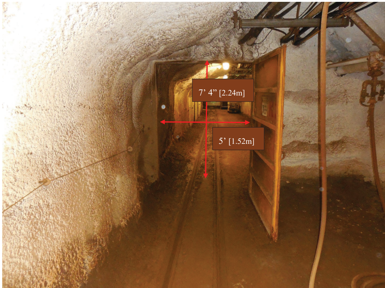
Figure 26: North Entrance Drift Access Door
